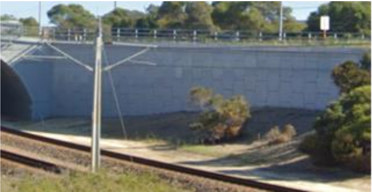
Figure 5 Image showing the steel barrier on top of the retaining wall protecting the rail corridor from vehicles travelling on the freeway
