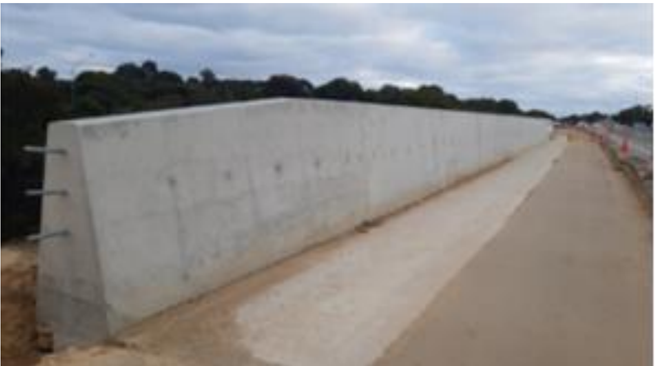
Figure 6 The steel barrier on top of the retaining wall has been removed and replaced with the concrete structure seen in the image above
